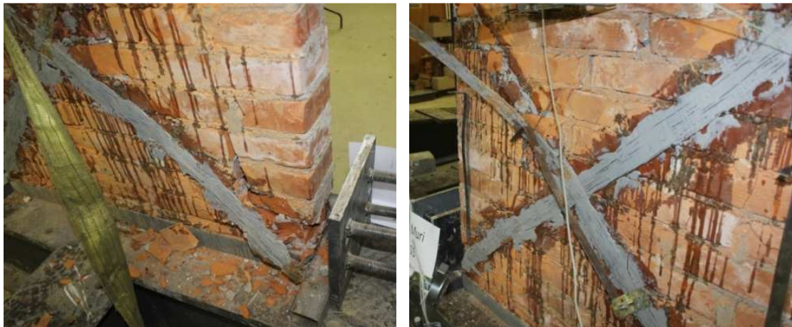
Fig. 10. Failure mode and delamination of GFRP
