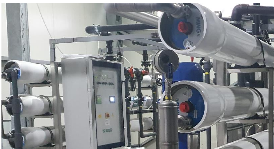
Fig. 1. Specialised Technological Component for Processing and Recirculation of Softened Water Required in the Research of Aluminium Alloy Plates Quenching Process
